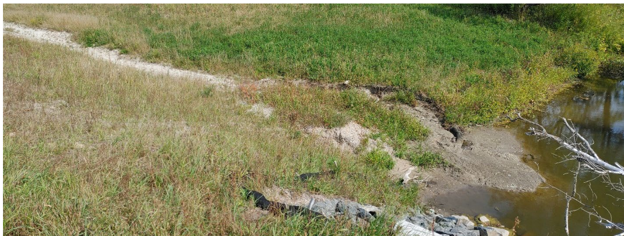
Erosion at North Cormorant River
